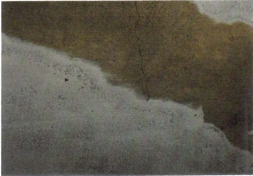
FIGURE 6: High Stress Area at Level 1, Willis Street Showing: - crack and its bridging by membrane - removal of membrane but no delamination
