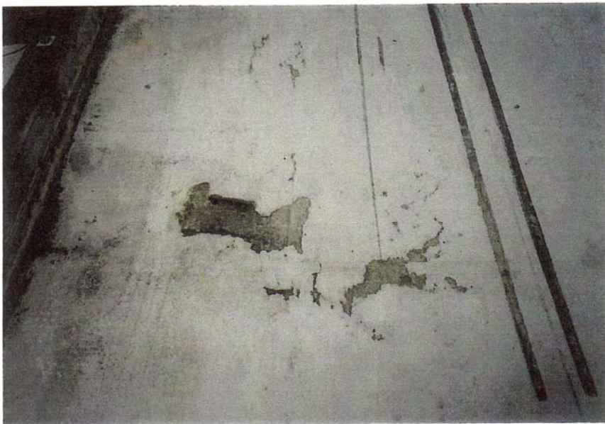
FIGURE 7: Delamination in Localised Area of Water Ingress
